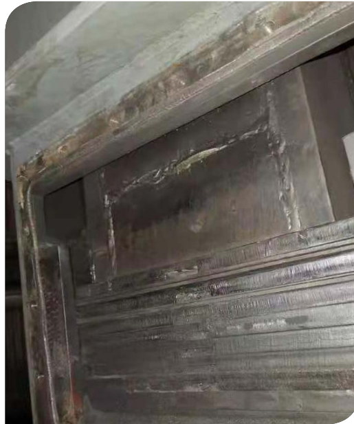
Coal pulverizer after transformation
